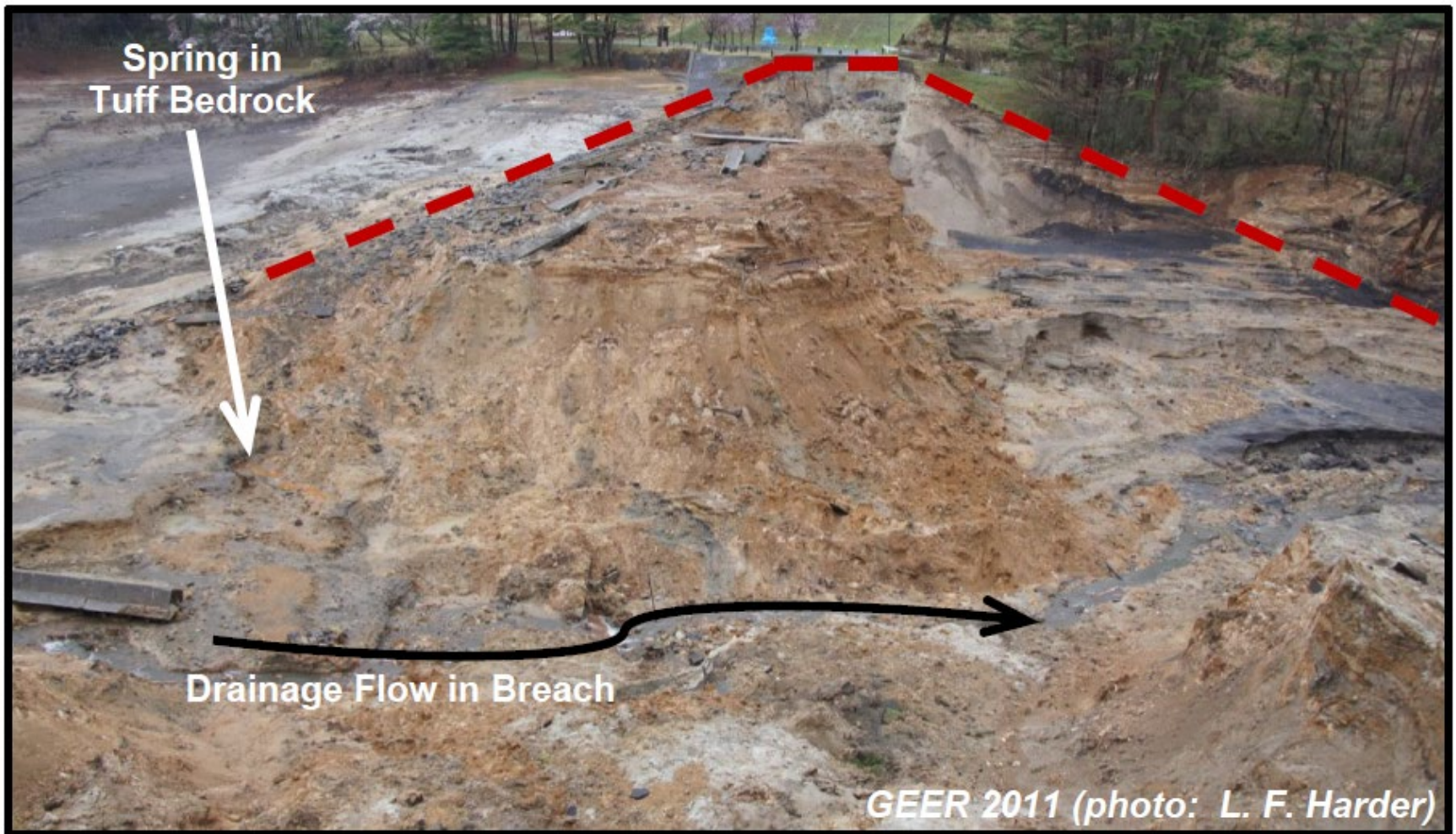
Figure 8: View of Breach in Fujinuma Main Dam from Right Abutment (N37.3014°, E140.1957°, April 23, 2011)
